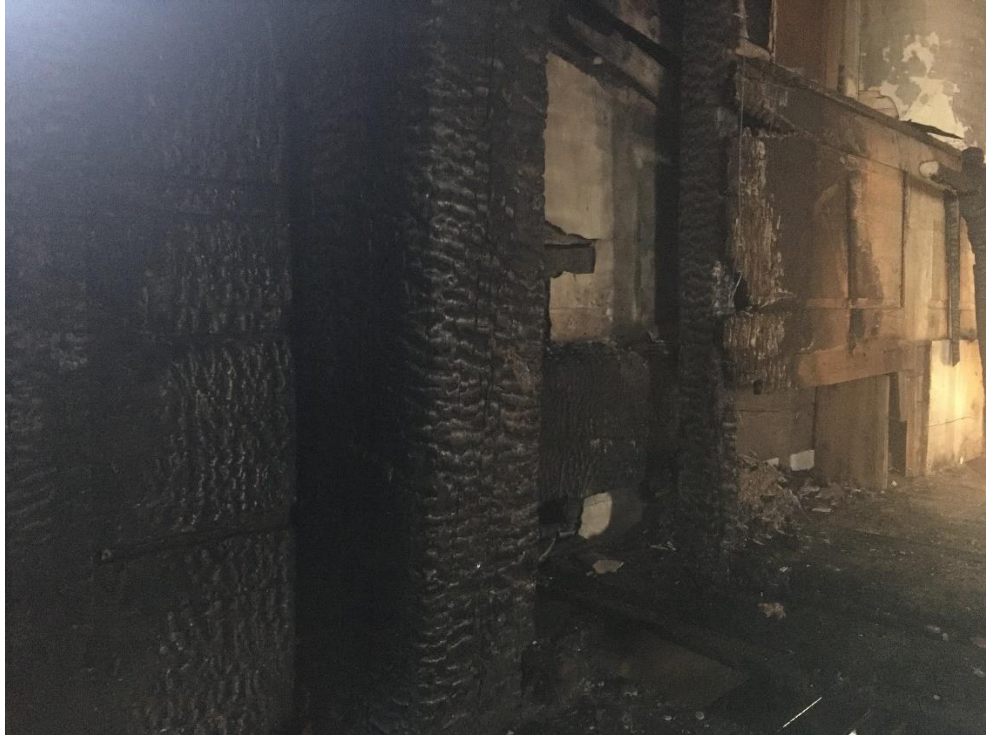
The north side's central bents' posts sustained the most fire damage and will likely need to be fully replaced if the removed charring reveals too much structural damage.
