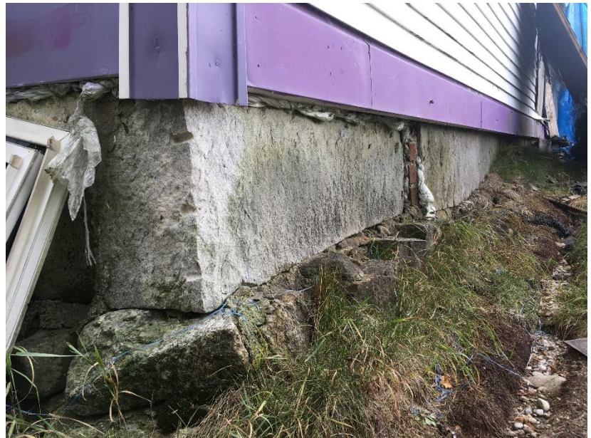
Condition of granite foundation at the NE corner.
