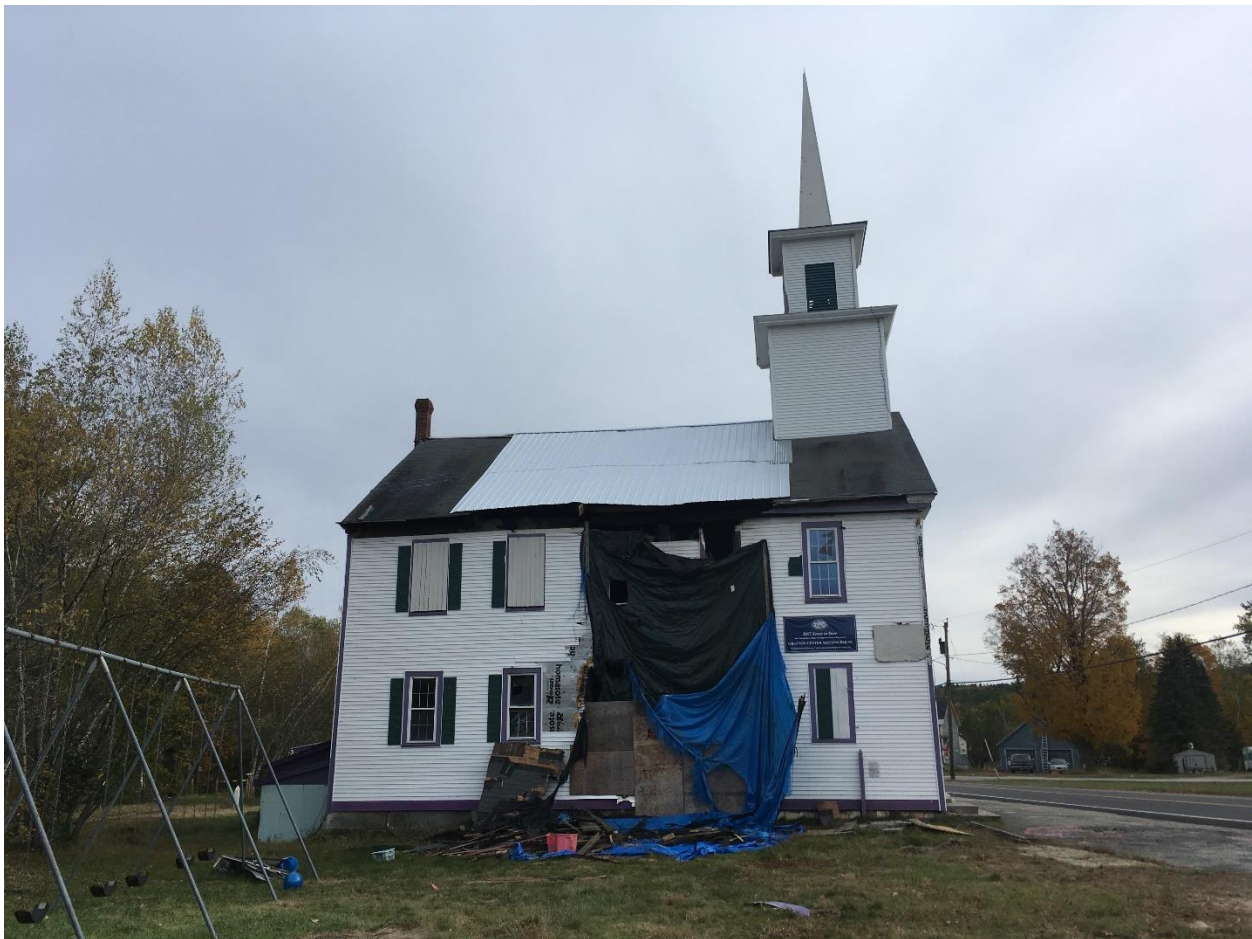
North elevation, showing the worst of the fire damage.
