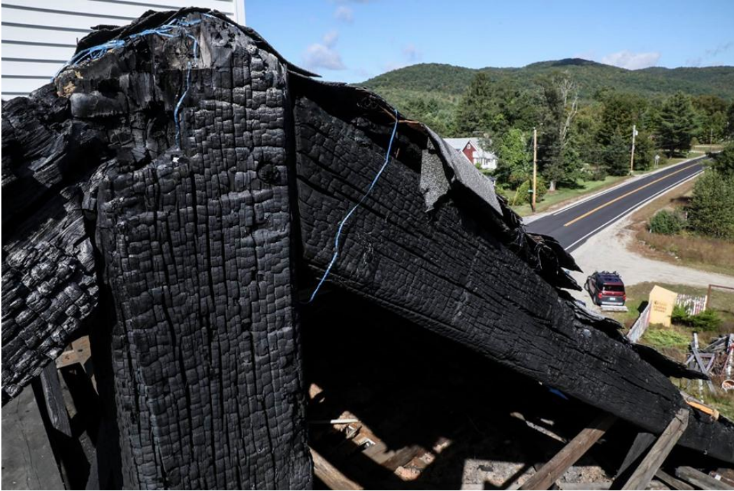
Close up of charring at a king post and rafter joint.
