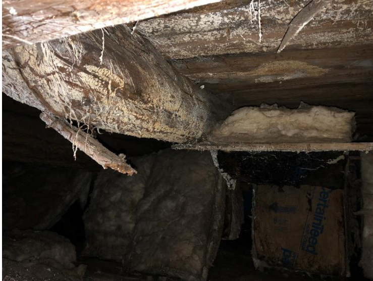
Undercarriage, showing fiberglass batting and mold growth.
