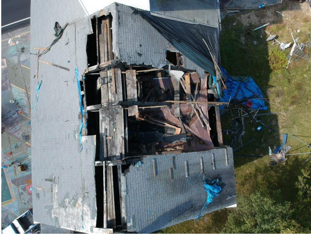
Aerial view of the roof with portions of the roofing removed. The middle bent is without a rafter, and is temporarily connected to the top plate with dimensional lumber.
