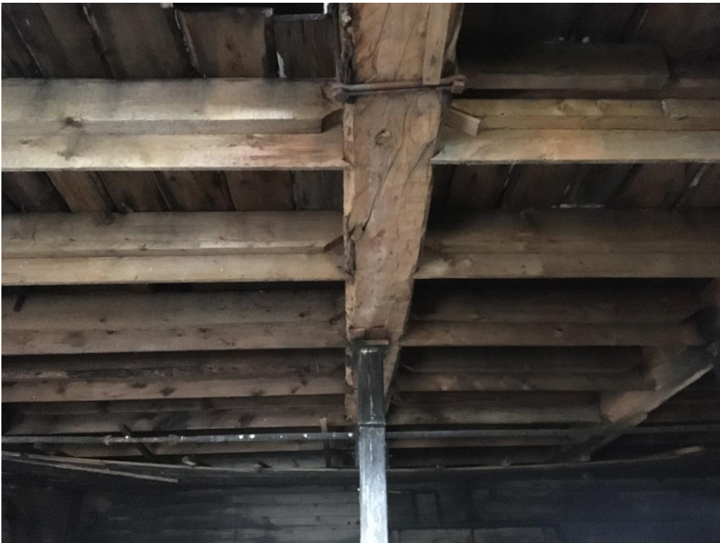
The second story floor system appears to be in good shape and should continue to dry out over the winter.
