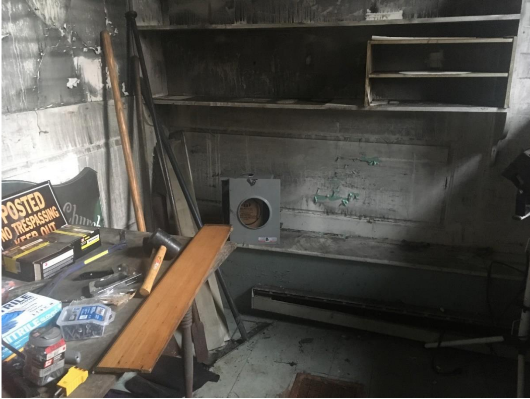
Paneling in the stair landing room at the SW corner of the first floor, showing paneling.
