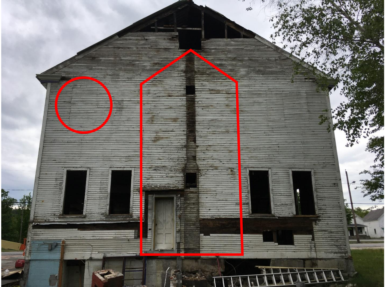
Rear elevation of the Meetinghouse, with ghosting of second story windows and rear porch outlined in red.
