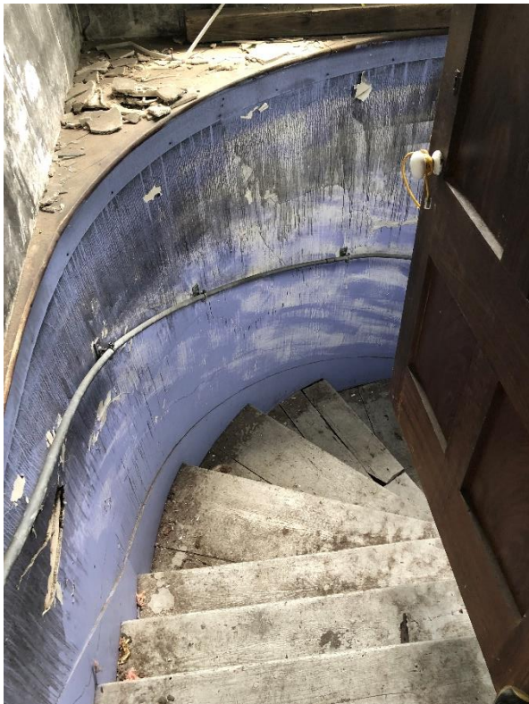
Above: the “coffin stairs” experienced heavy fire damage. Left: the SW spiral staircase survived the fire.
