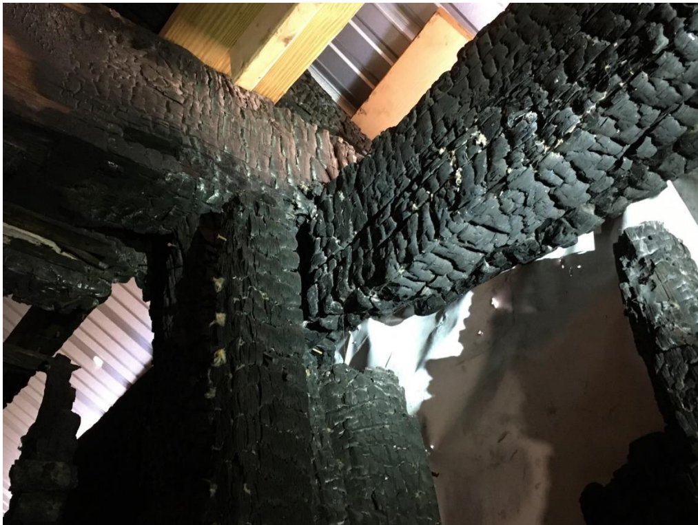
Close up of a joint at a central bent, showing the extent of charring and weakened joinery.
